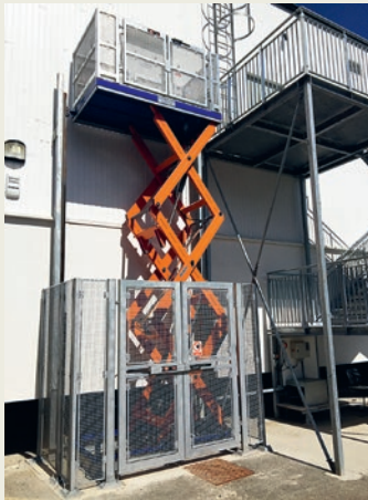
Goods and freight lift
